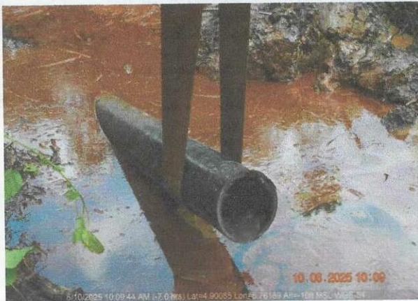
Fig 2 Showing the severed point at 6" Ajatiton 1L/S
